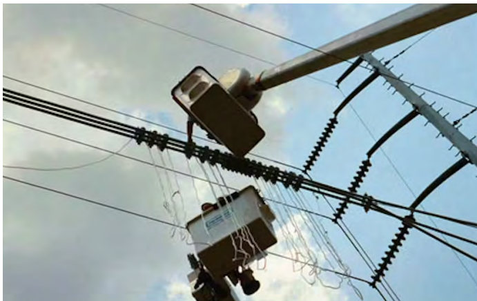
Crews prepare to install spacers at 20 foot intervals by using string to measure the distance between each spacer, an easy and accurate method of installation.
