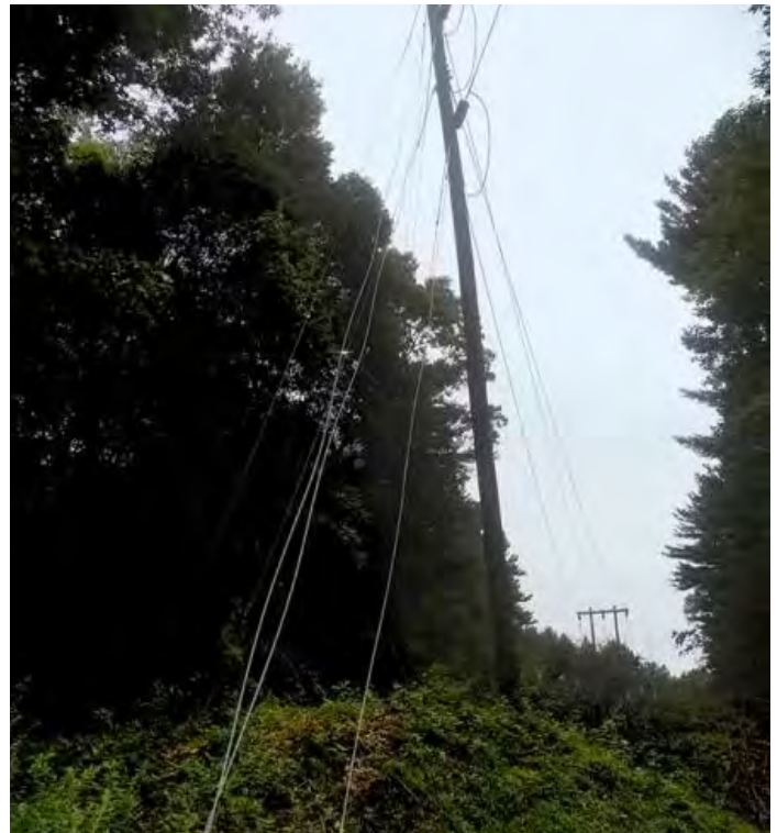
This typical dead-end structure is leaning and needs maintenance.
