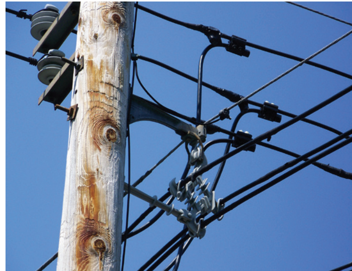
Figure 7 – IPCs installed on a covered conductor in the field.
