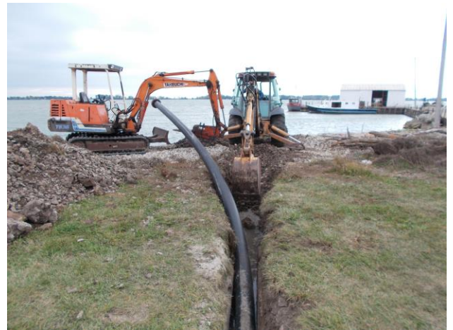
8-inch HDPE pipe installed on each shore landing to pull cable through.
