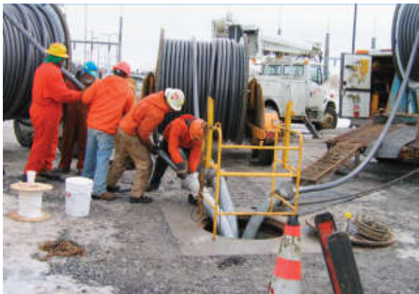
Three 115Kv Cables Installed in one Conduit.
