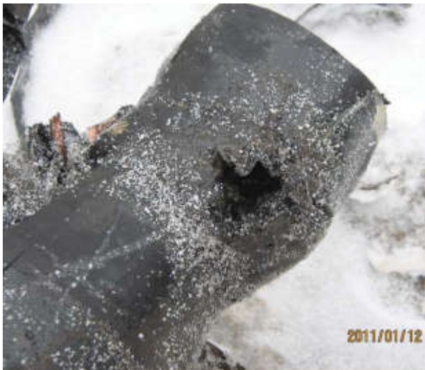
Failed 69kV XLPE cable removed.
