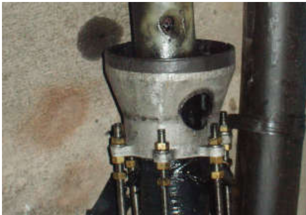
Failed termination that was replaced.
