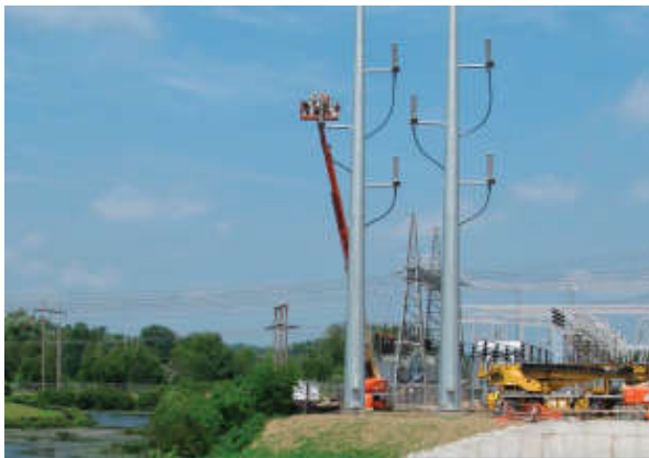
90 Ft pole with completed terminations.
