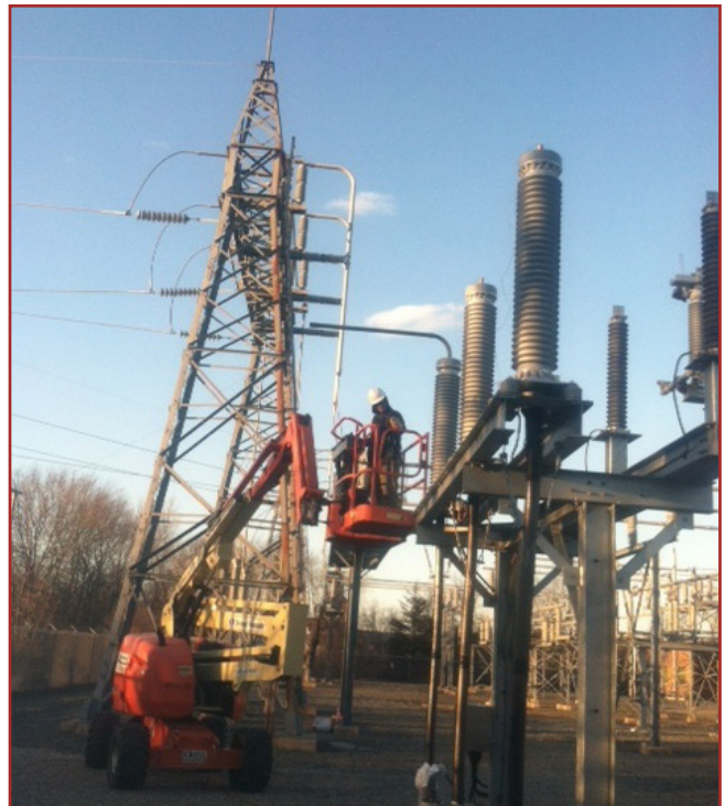
Acceptance test being completed from the switch yard side of the circuit run.
