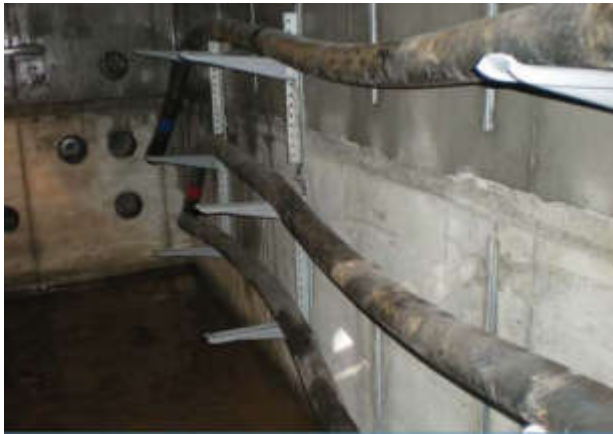
Existing cables in vault to be spliced.
