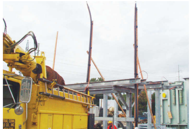
Cables Ready for Termination
