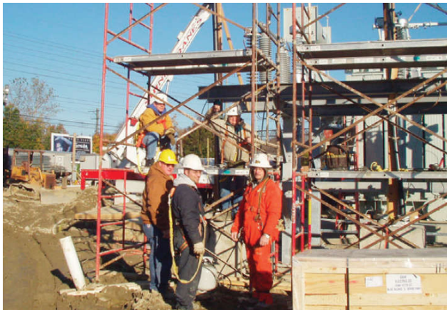
Cable Termination Scaffolding
