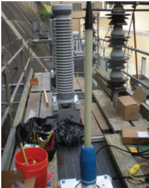
Termination with stress cone and finished termination.
