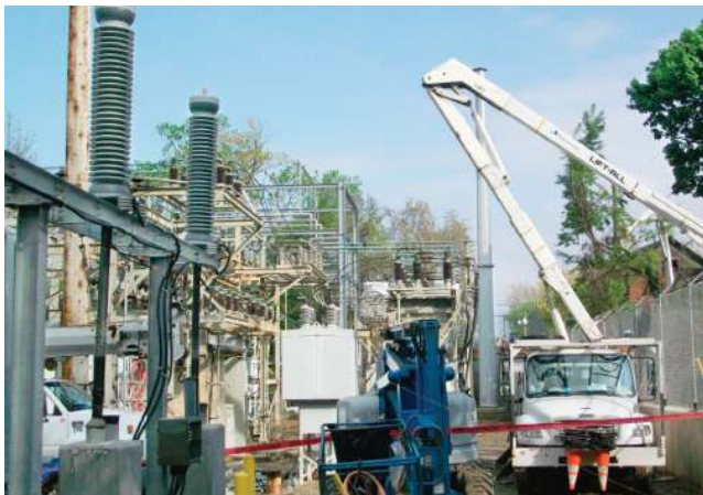
Making terminations within substation.
