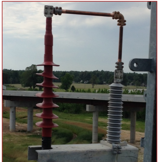
Termination connected to lightning arrester with 1-1/2" IPS copper bus tubing. Jumpers from the overhead 69kV line were attached to the NEMA 4 hole pad on the top of the termination.
