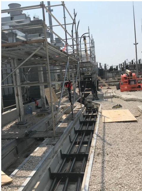
Cable installed in concrete trench
