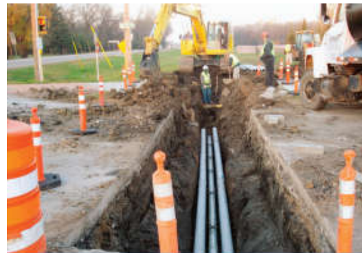
Open cut across four lane street. Conduit laid and street repaired by Ernst Trenching.
