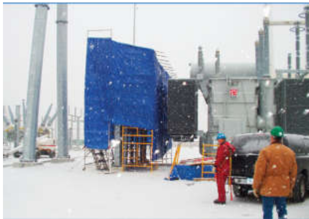
Cable Termination Shelter.
