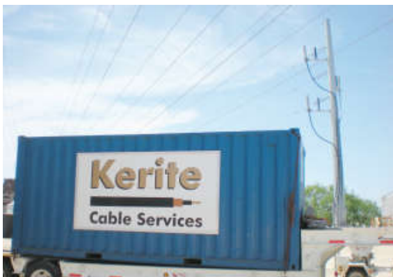
Three completed G&W terminations on 70 ft. riser pole.
