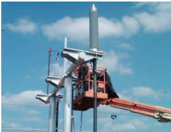
Completed HV termination
