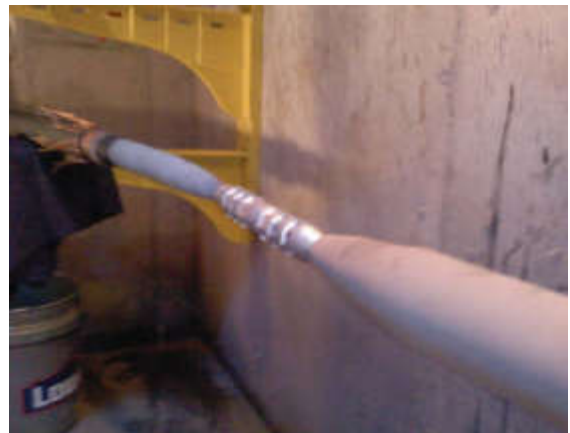
Splice between 138kV EPR and 69kV XLPE cables
