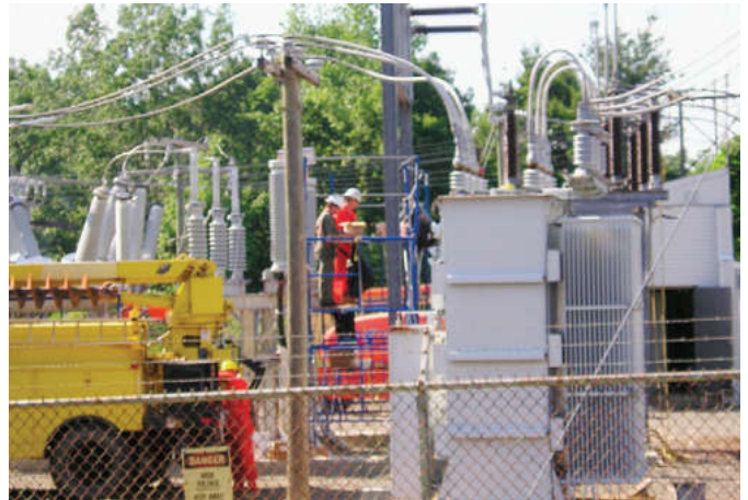
Cable Termination Structure
