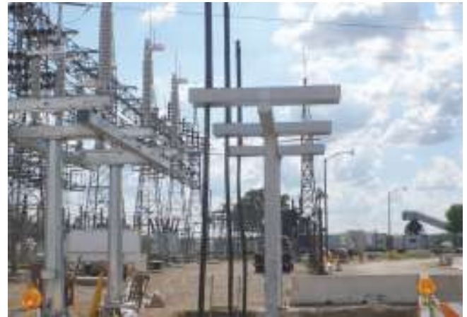
HV cables installed on terminations structures.
