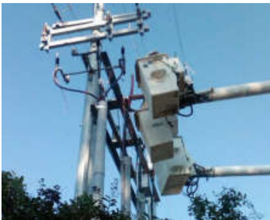
69kV heat shrink terminations.
