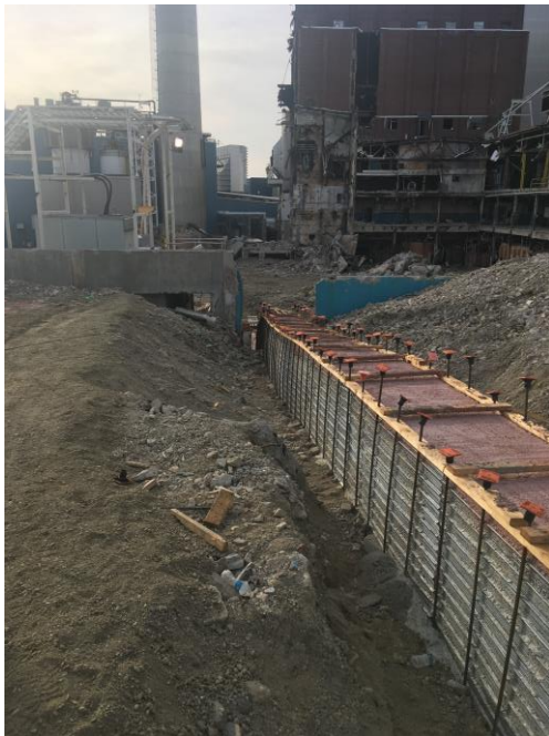
Concrete encased duct bank
