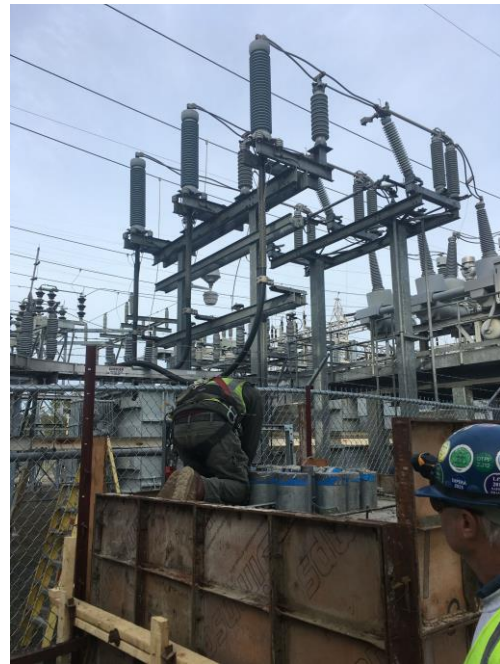
115kV termination riser structure
