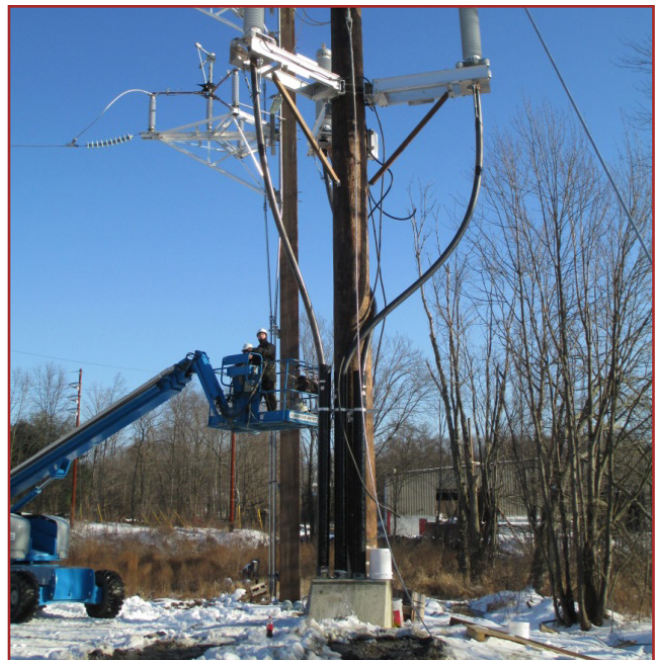
3- G&W PAT 140 installed on Riser Pole
