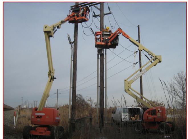
KCS along with Anderson & Wood technicians work in two separate teams to complete G&W PAT 119 terminations on riser poles.
