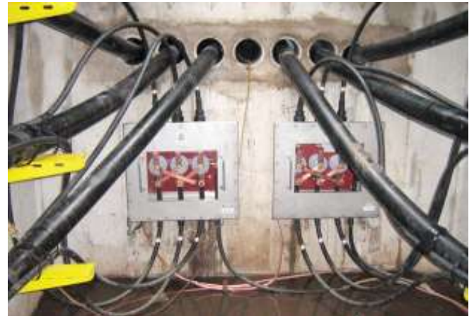
Cross bonding boxes in vault.
